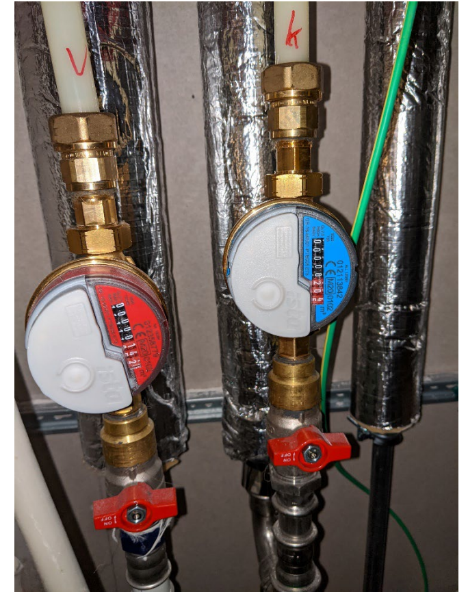
Hot and cold water
